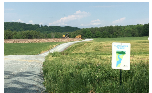
Above: Clean Water Project Sign displayed on the path to a Best Management Practice construction site.
